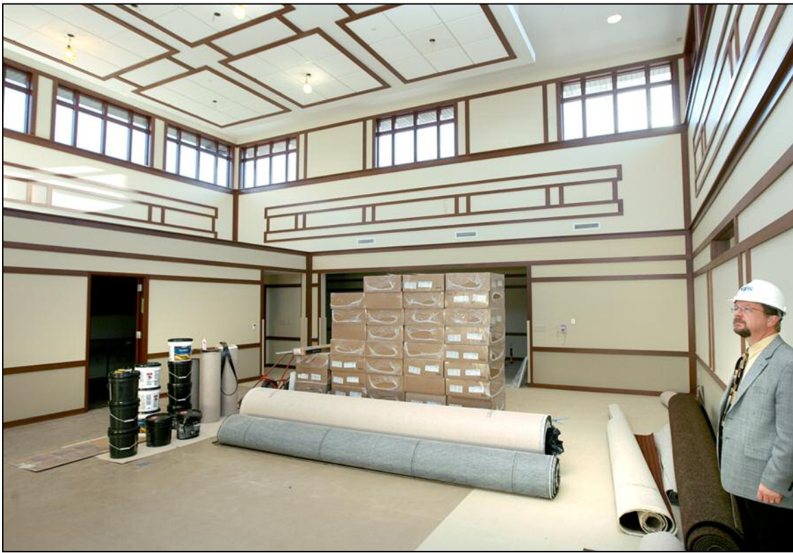
Bro. Mark Strautman, Three Pillars President & CEO, looks over the progress in the therapy room of the new rehab center. The workmen are very near completion, making way for the installation of the new state of the art equipment to be installed.
