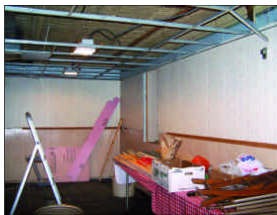
The rain was so heavy in Columbus that the force of the runoff from the roof caused the downspouts of Columbus Lodge to come off, allowing rainwater to flow down the fieldstone walls and perk up through the basement floor, lifting tiles, soaking the carpet, walls and insulation. Ceiling tiles were also ruined in the process. – Photos by Bro. Bill Barnes
