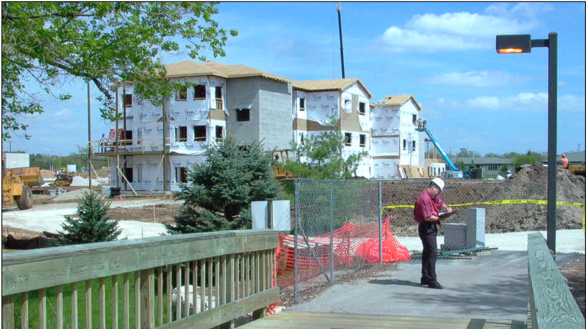
The walls are up, the roof is on and interior partitioning has begun on the three story portion of Three Pillars' new Catered Living Residential Care Apartment Complex on the Fraternity's senior living campus in Dousman. Brother Jerry Hoepfner (on bridge at right), Three Pillars' Director of Environmental Services, takes a phone call in his role as logistics coordinator between the construction company and Three Pillars. A spring 2006 completion date for the $14 million project is planned. This picture was taken May 10. – Photo by Wm. Stonecipher
