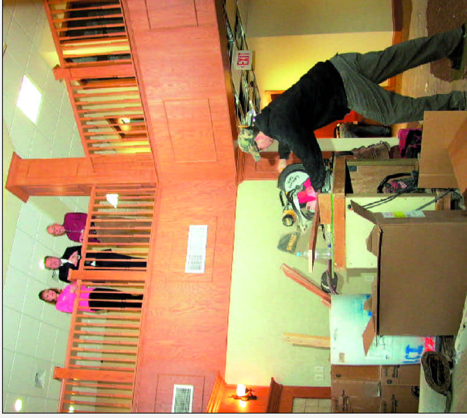
Carpenter Abe Rozmarynoski worked at putting the finishing touches on the main entry area of the Compass Point Catered Living facility in early February. Watching from the balcony were Don Lintner (right), a resident of the Masonic Village on the Square, Jessica Kolsch, Campus Housing Manager, and Bryan Polinske, Administrator of Senior Living Services at Three Pillars. It is planned that residents will begin moving in during early March.
