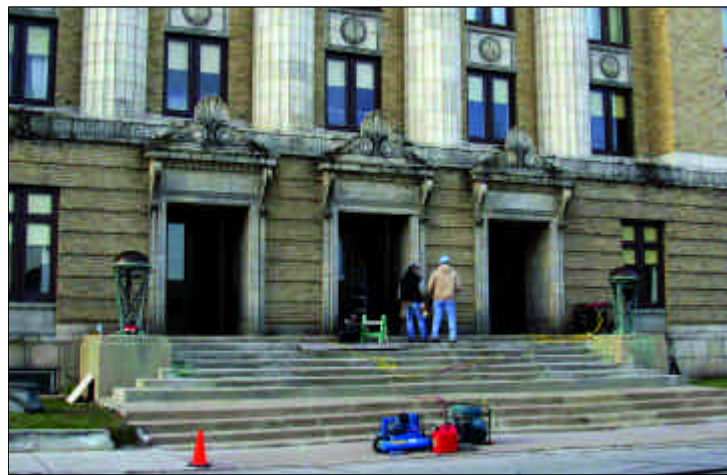
As part of the arrangement between Universal Studios and Oshkosh Lodge for using the building for the filming, the steps were repaired (work shown above) and bank-like doors were installed to replace the original ones. The particular series of scenes involving the Oshkosh Masonic Center building recreates a bank robbery that actually occurred in Racine, not in Oshkosh. The lodge also received payment for the use of the building as a movie set.
