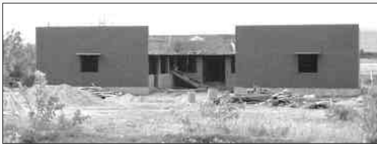
This is the Ciriacks Girls House as it appeared in August of this year. It will house 48 orphaned, poor and unwanted girls aged 6-18 in Madurai, South India. The 5,000 sq. ft. building was made possible by a donation to fulfill a dream by Brother Sam Ciriacks, a member of West Bend Lodge No. 138.
